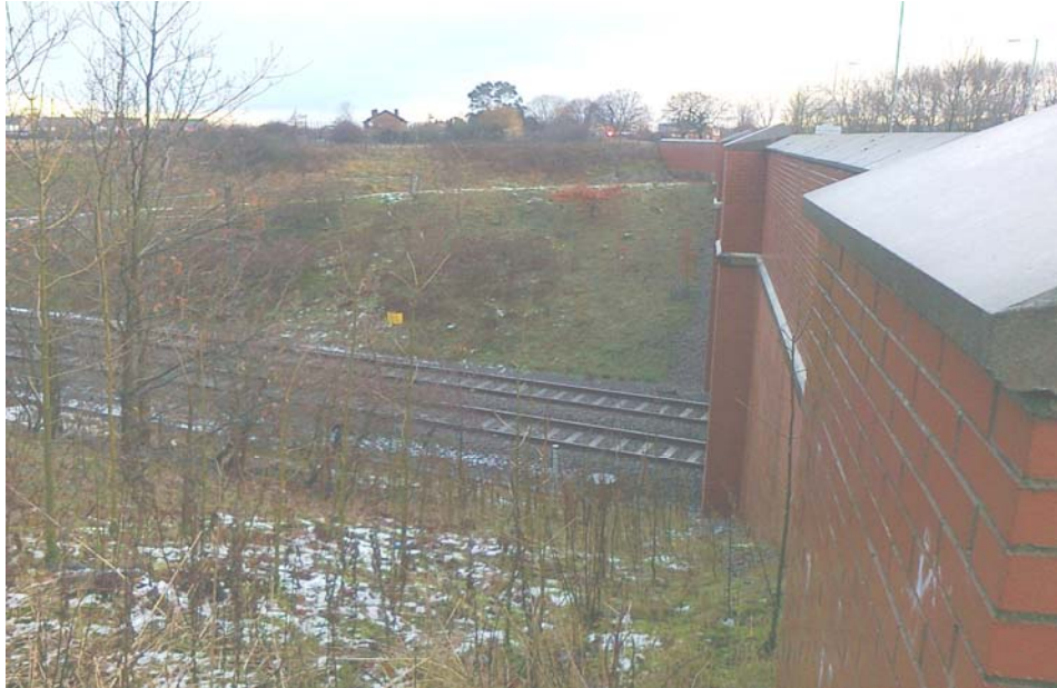
View on the west side of the existing structure showing the bund and the south spur
